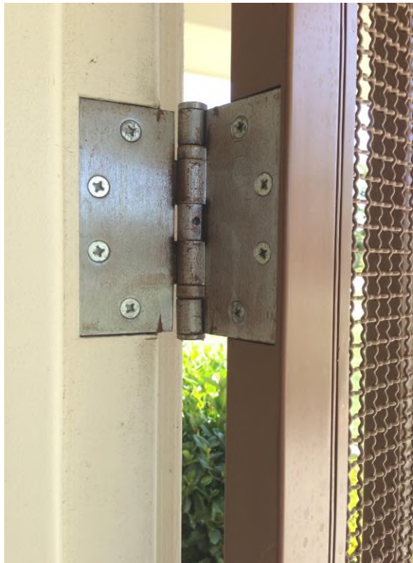
Properly Installed Gate-Frame Hinge
