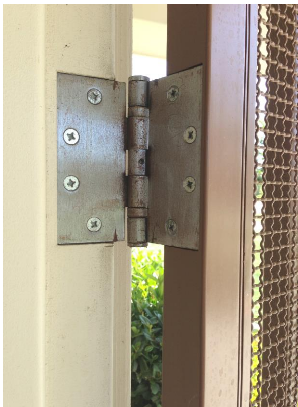
Properly Installed Gate-Frame Hinge
